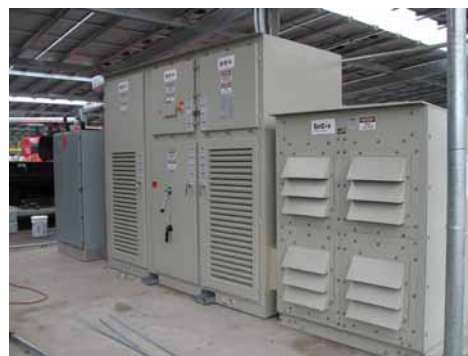
Grid-tie inverter and associated equipment
