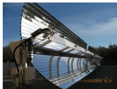
Photo 2: Solar Mirrors and PV arrays
